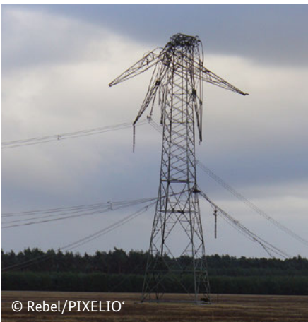
Storm damage caused by Hurricane Kyrill in 2007
